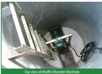
Top view of Muffin Monster Manhole
